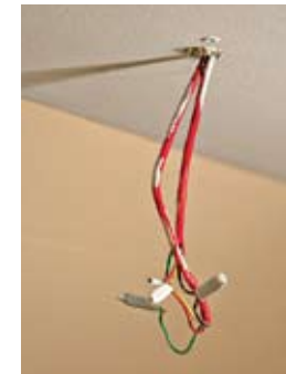
These exposed wires were a real shocker.
